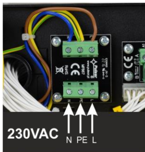
PCB Power Board in the Patch Panel
