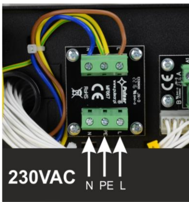
PCB Power Board in the Patch Panel
